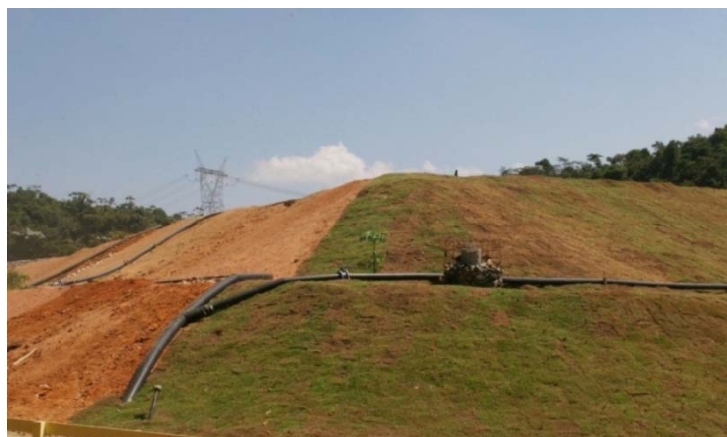
Figure 2– Example of Transmission Pipeline – Adrianópolis Landfill/Brazil
