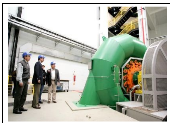
PCH Esmeralda-RS com 22 MW
